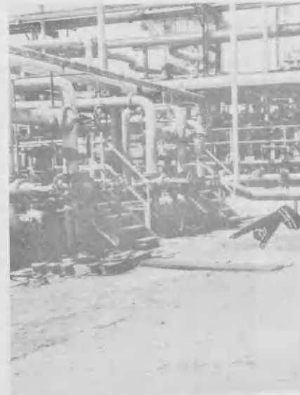
A sure sign of bad housekeeping is the piping, and even shoes and gloves. This is north of the central pipe-alley. Muestra sigur di descuido ta e lugar di zapato y handschoen. E lugar e zuid-van pipe-alley den
